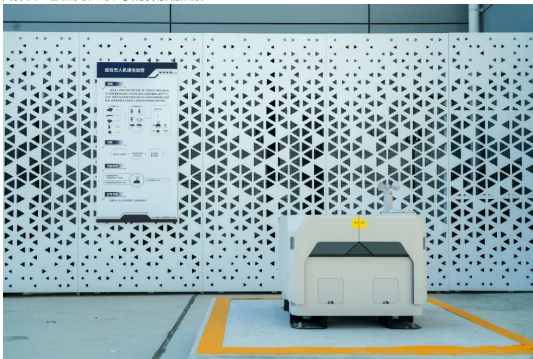
▲变电站实现巡检无人机通信加密
